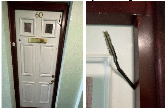
f) Flat 60 – Access not gained but it appeared that the cold smoke seal was partially detached.
