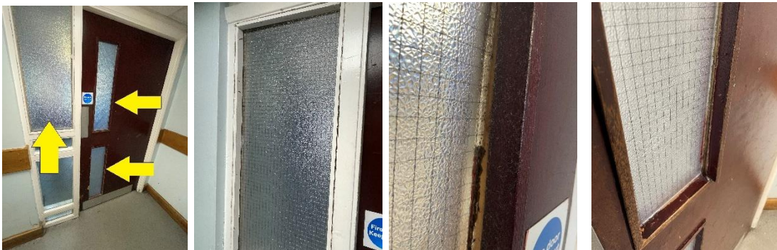
15) Communal door from lift lobby to stairwell, 3 x Fyberglaze GRP panels are loose and require refixing. Upper panel in combination frame is poorly fitted and loose. Upper panel in door - beading / panel not secure. Lower panel moves / not secure.
