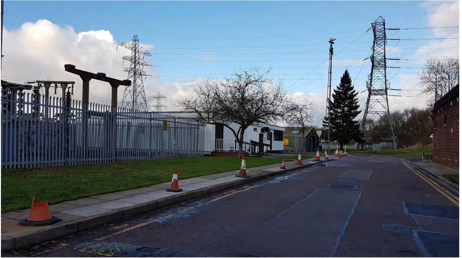
View of entrance to substation off Greenfield Lane
