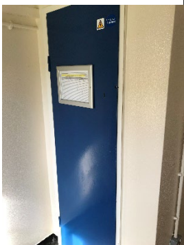
(steel door block 19-24) no intumescent strip or smoke seals
