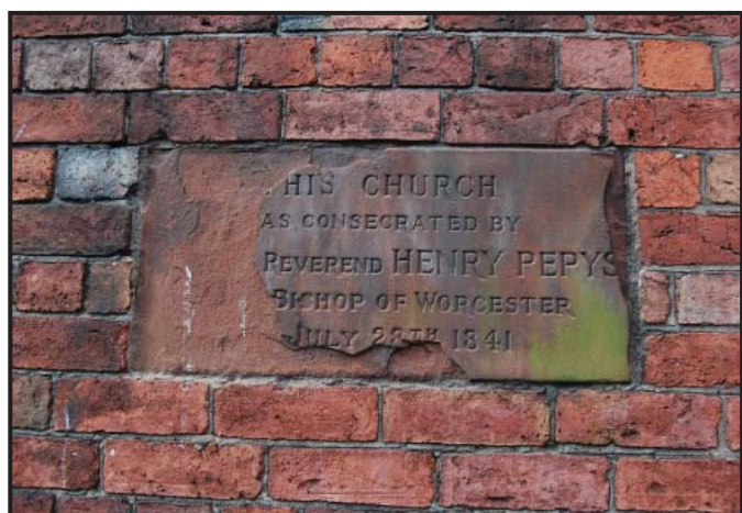
Plate 57: Crumbling dedication stone, Christchurch.
