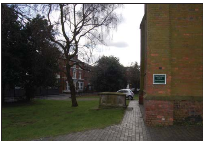
Plate 56: Moss/lichen on Christchurch brickwork.
