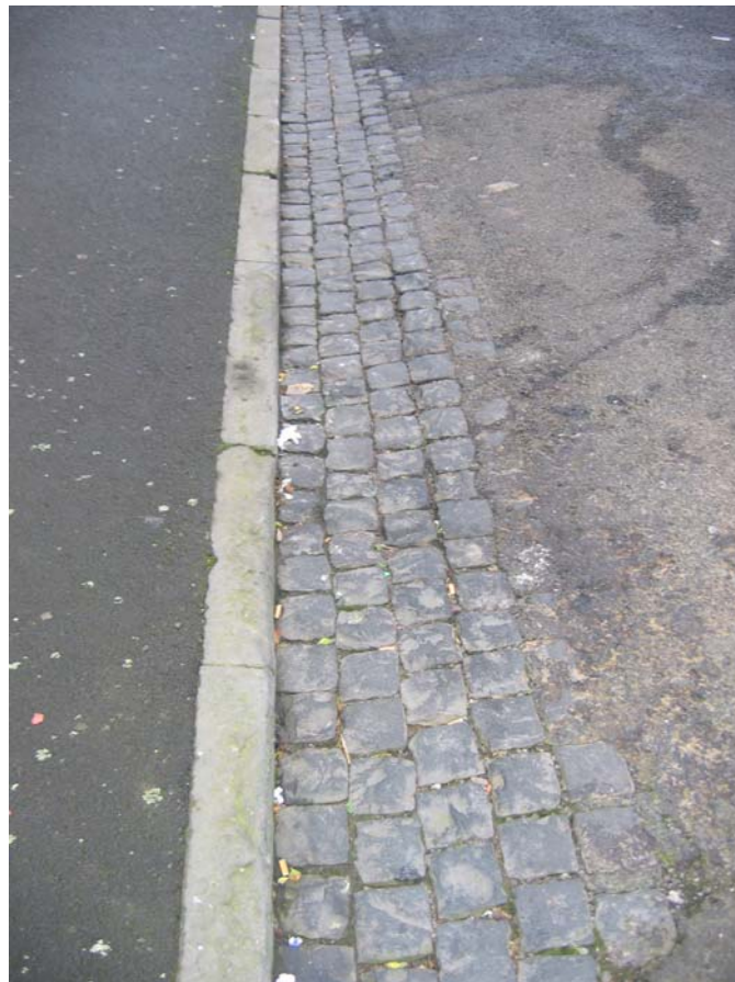
Plate 2: Kerb detail on St. Alban's Road
