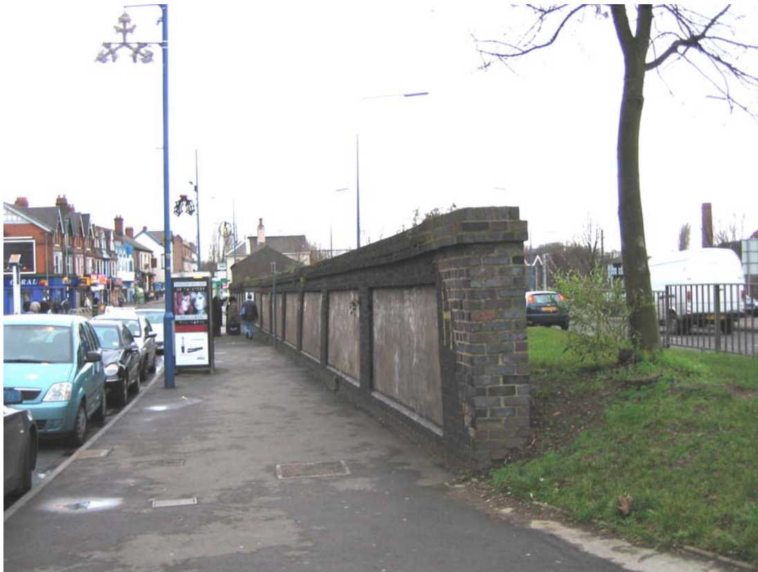
Plate 28: Former railway yard wall, looking northwest along High Street
