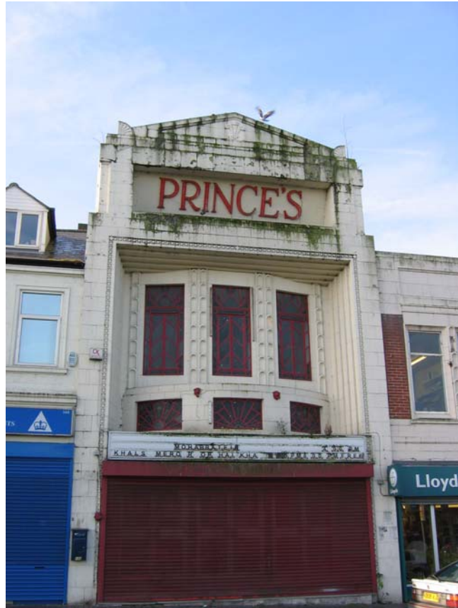
Plate 43: Façade of the former Prince's Cinema, showing state of disrepair
