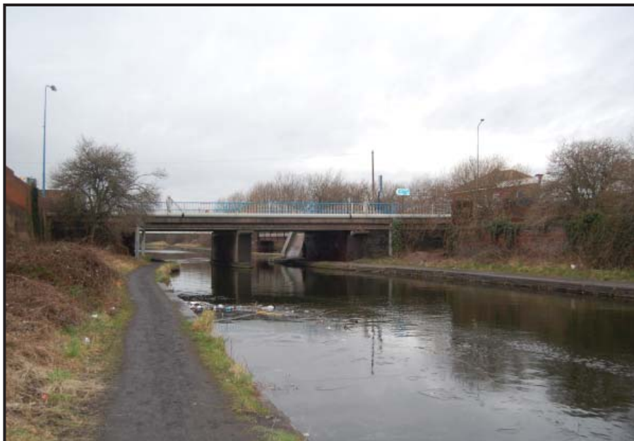
Plate 47: Rubbish in canal.
