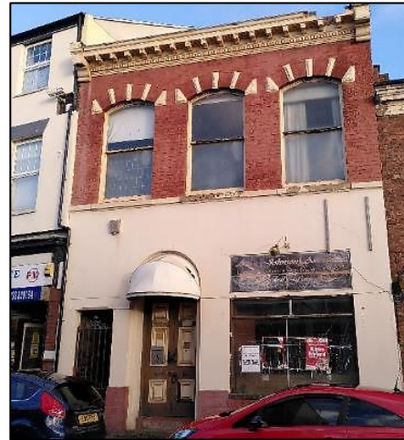
Figure 80 Poor quality signage, Lower High Street.
