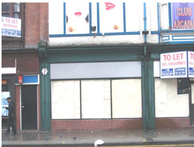
A typical traditional shop front.(unfortunately infilled with modern glazing and brickwork).
