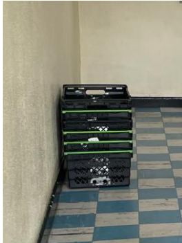
c) Block 106-114 – Asda home delivery baskets in ground floor means of escape.
