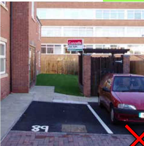
Poorly delineated car parking located too close to habitable rooms, in a sea of hard surfacing .
