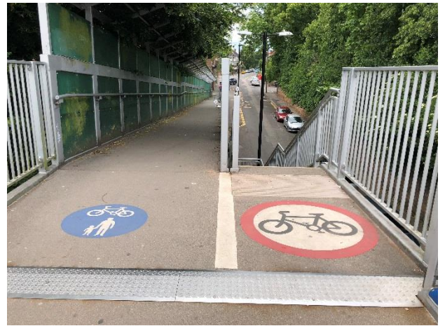
Photo 4 – Existing pedestrian and cycle bridge crossing the ring road between Hill Street and Upper Hill Street
