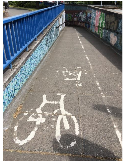
Photo 4 – Existing cycle provision under Penn Road Island, but provides an unattractive route
