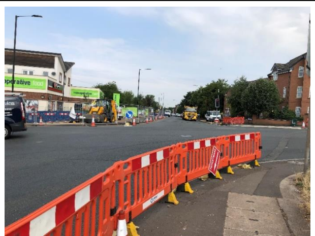
Photo 6 – Current works at junction of B4152 / Lichfield Road / Brownhills Road. Constrained geometries and lots of HGV movements
