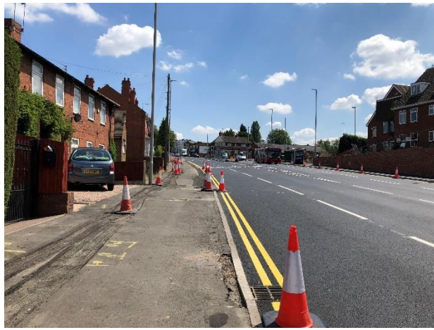
Photo 3 – Wide staggered signalised junction at A4101 High Street Pensnett / B4179, which has recently had improvement works
