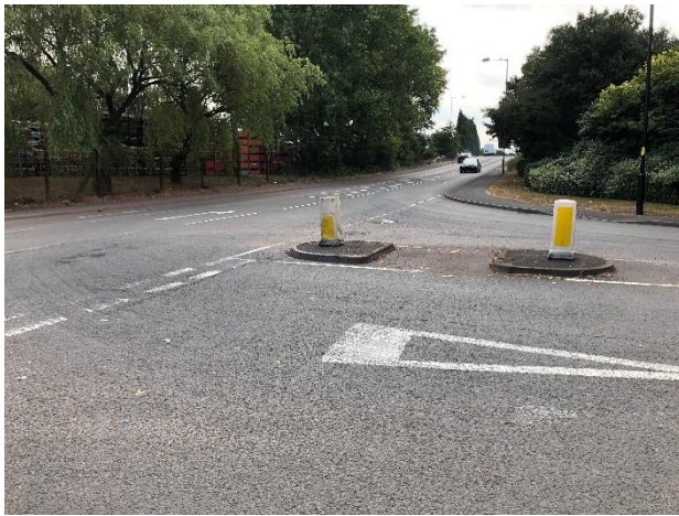
Photo 3 – High traffic flows, speeds and steep gradient on approach to canal bridge on Stubbers Green Road
